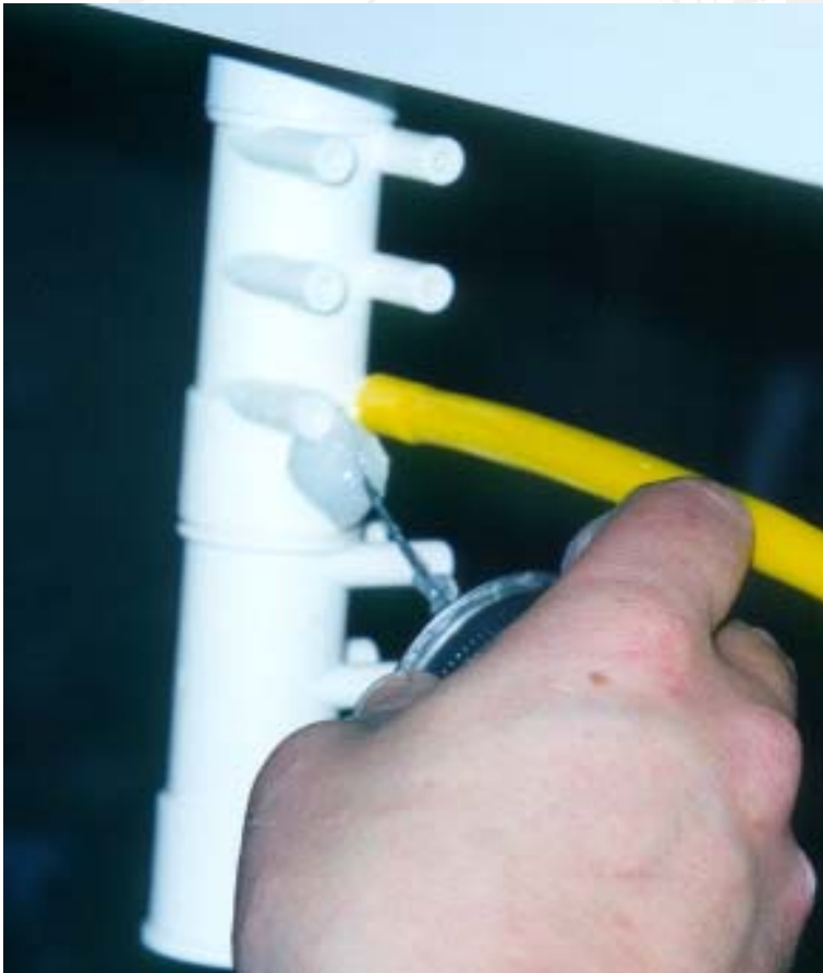
Above: Always glue the manifold not the pipe - Take care not to block any spigots with glue - especially when glueing the stop end
